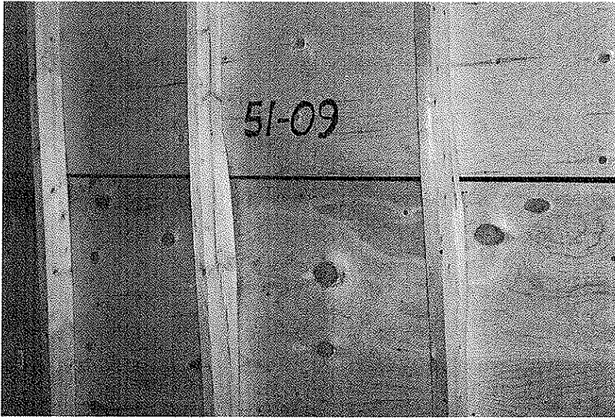
Figure 7 Studs split along the unblocked horizontal joint with 100 mm nail spacing.
