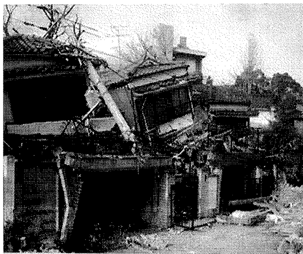
Photo.6 - Collapse of the second story. The first story was a garage of reinforced concrete.
