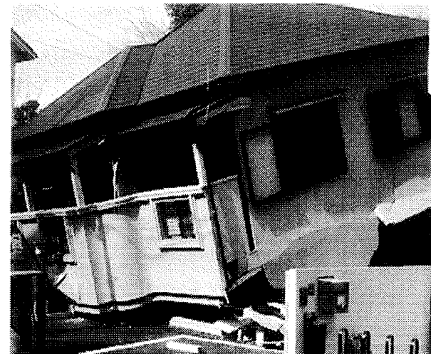
Photo.4- Collapse of newly constructed house. The first story was garage and the displacement of shear wall was eccentric.
