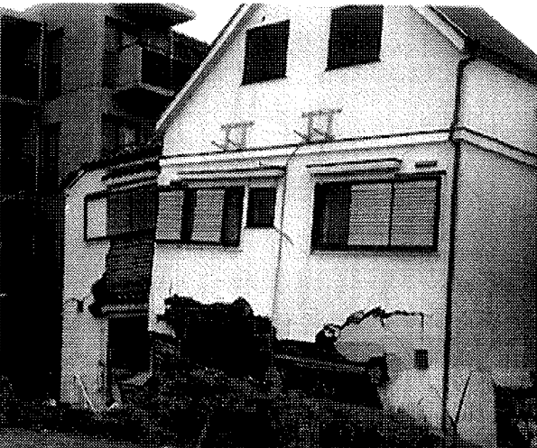
Photo.5 - Collapse of the first story. The third story was added afterwards.
